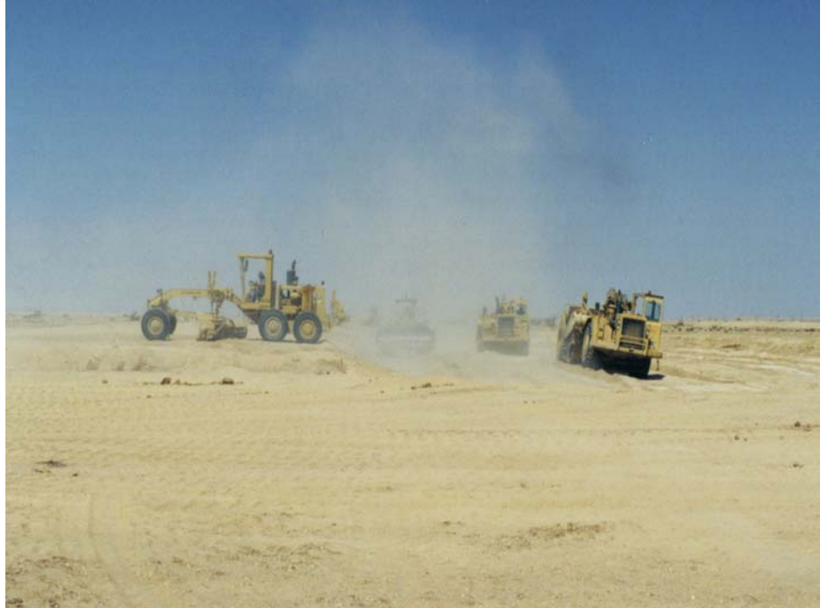
Situations requiring dust suppression are identified through daily field inspection (part of internal monitoring programme)
